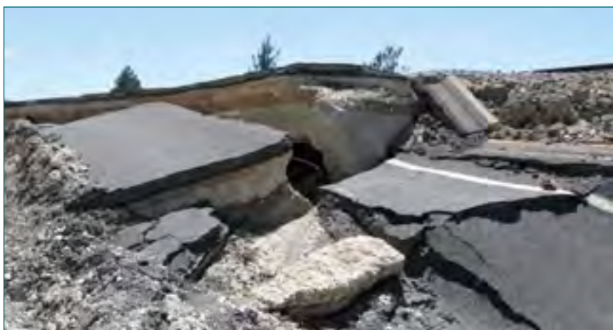
Road damage after the 7.8-magnitude Kaikōura earthquake. Photo: Scott Hammond/Stuff
